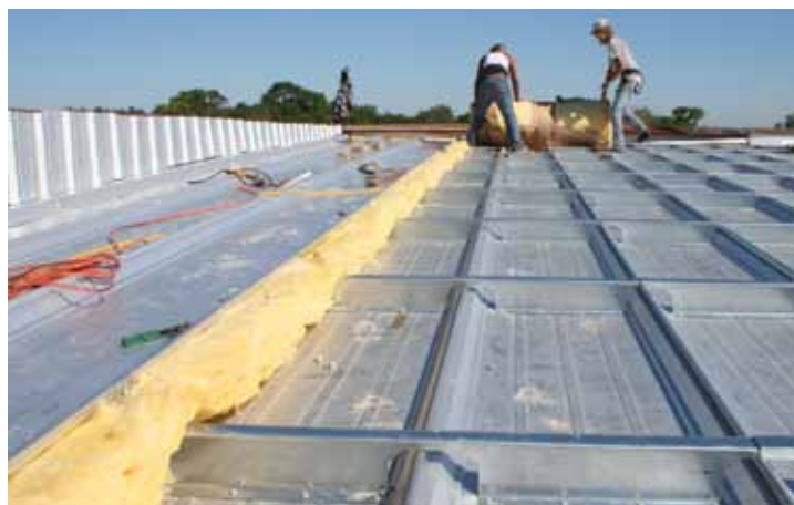
A trapezoidal standing seam roof being installed over an old trapezoidal standing seam roof with optional insulation.
