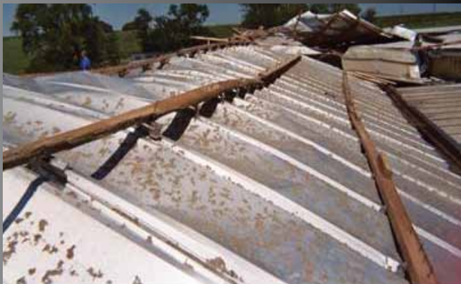
Wood framed supports add no strength nor support for a new roof.
