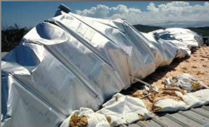
High SSR clips allowed wind to tear this roof apart.
