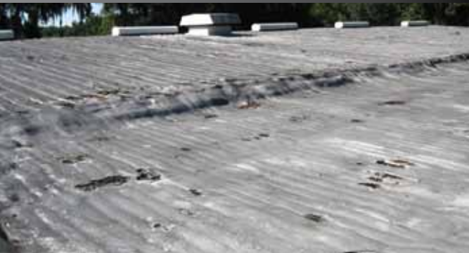
Coatings fail to stop problems permanently.
