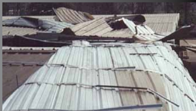
Hat Channel failure showing substandard re-roofing system.
